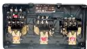
Interior View of MK1 SASD
