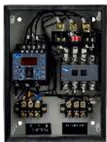
Interior View of MD Starter+ DOL Starter
